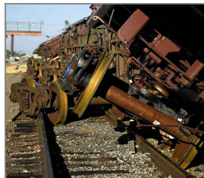
Hurricane Michael pushed a train off its tracks in Panama City, Florida.
