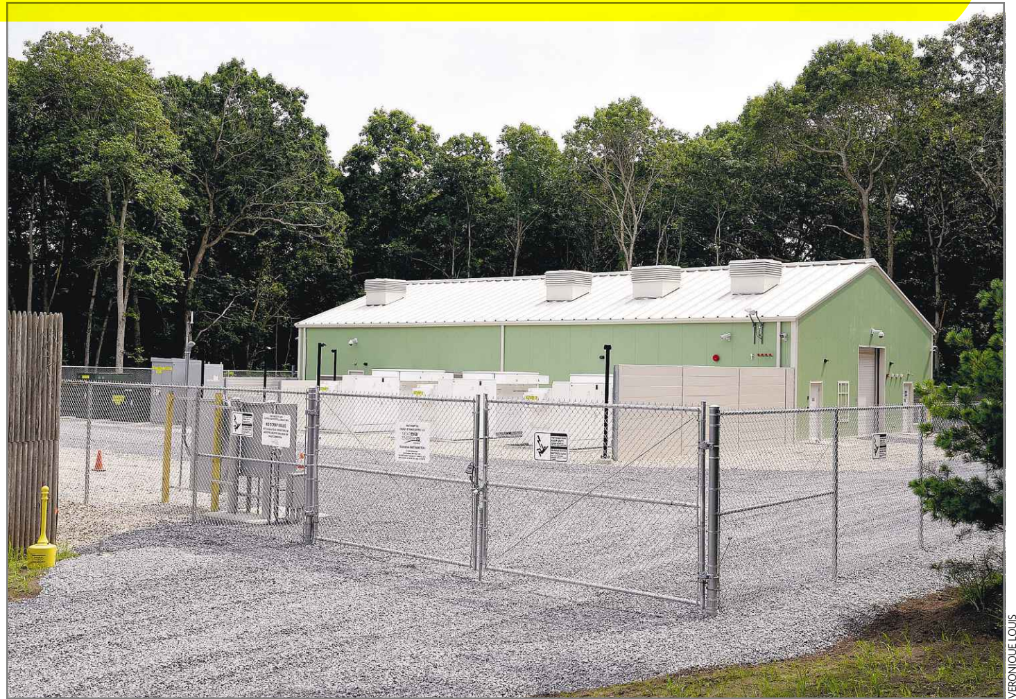
The 5-megawatt battery storage unit, at a LIPA substation in East Hampton, will improve system reliability in the Hamptons.
