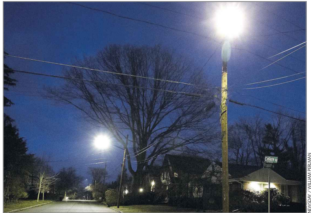
Great Neck has installed about 800 LED streetlights and says they may halve the village's electric bill.
