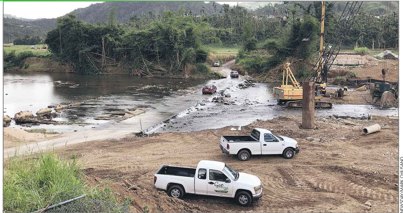
About 40 miles from San Juan, crews are just beginning to replace a bridge that was washed out in Morovis, in north-central Puerto Rico. Above, vehicles drive across a riverbed platform on Jan. 20. The far end of the lost bridge is seen at upper right.
