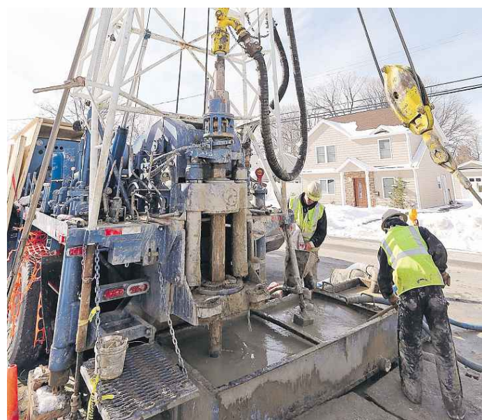
Investigating groundwater contamination in Bethpage.
